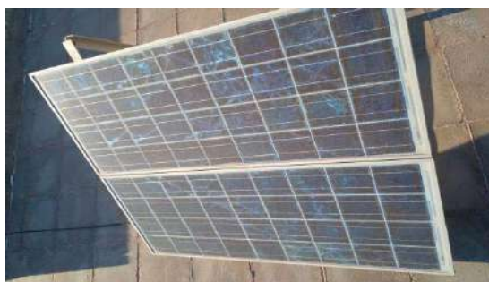
Fig .6 PV panel
